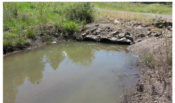
Figure 1: Pooling at CMPs [3]
